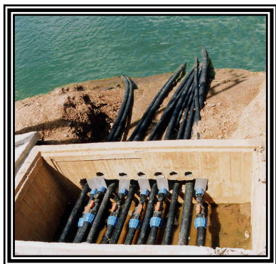
Compressed air pipes entering the reservoir
